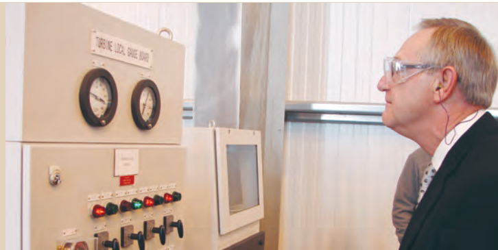
Marlboro Electric's President & CEO Bill Fleming observes all of the switches on the turbine gauge board for the steam generator.
