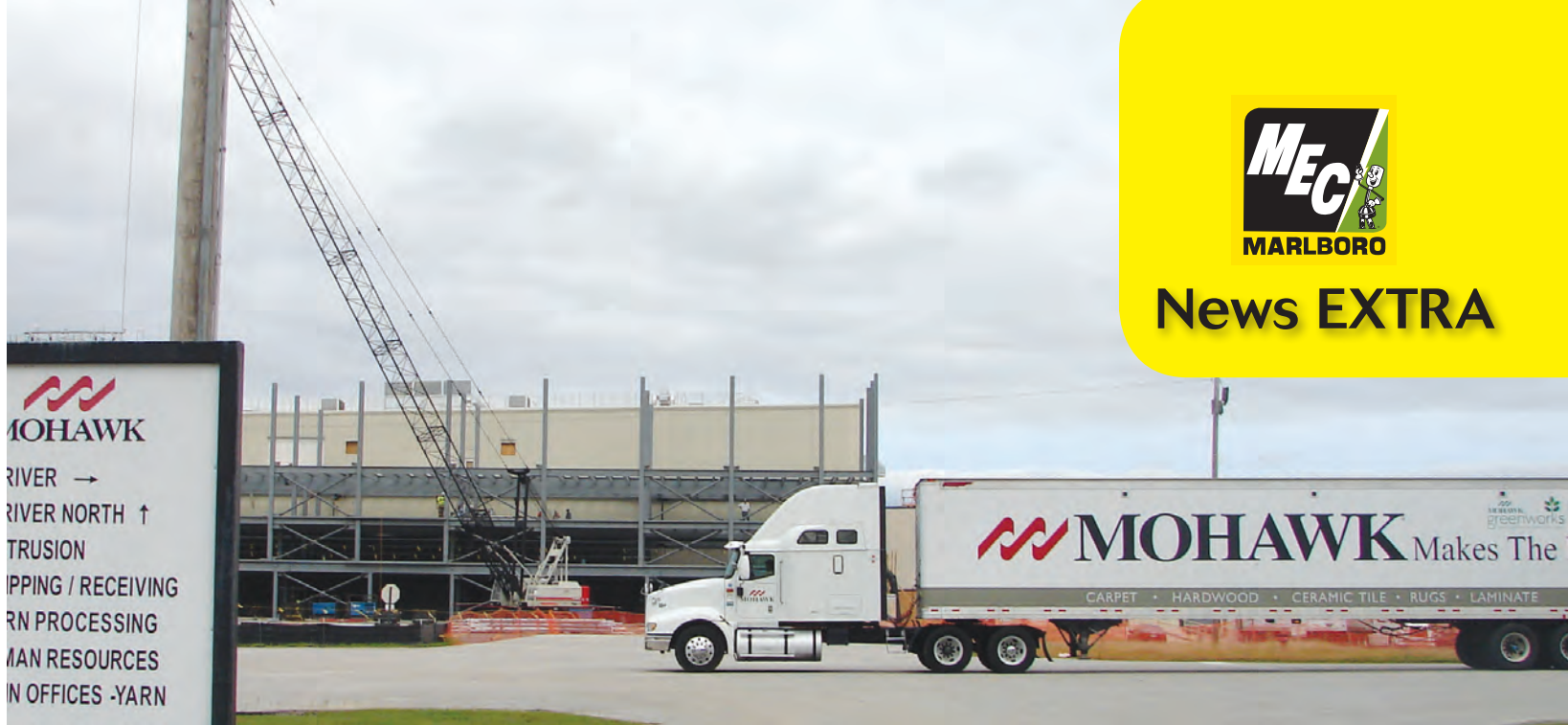
Mohawk Industries expands their facility on the Bennettsville property served by Marlboro Electric.
